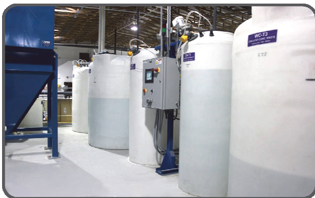
Fully-integrated waste management system
